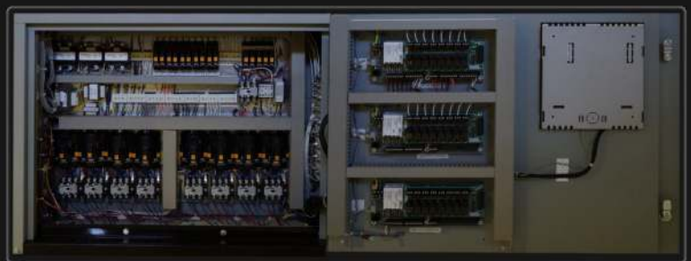
A PERFECT ARRANGEMENT OF ELECTRIC COMPONENTS
